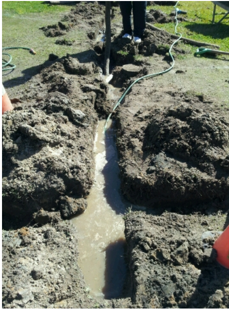
Photo taken August 2012 of a repair to a subsoil drain near Bissett Croquet Court
