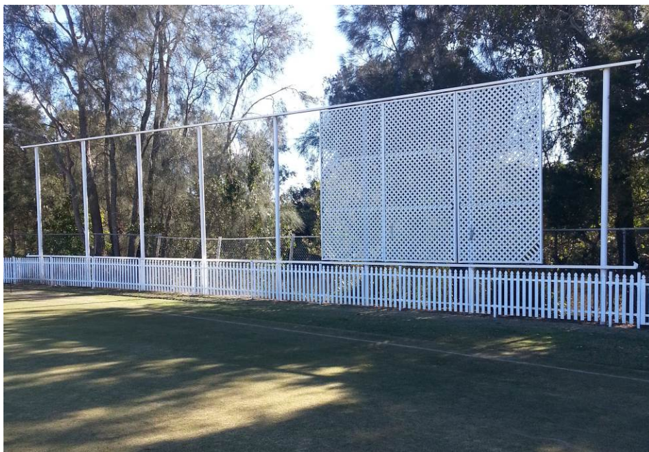
Photo of sight screens at the northern end of the oval taken 7 June 2016 after they were repaired and painted.
