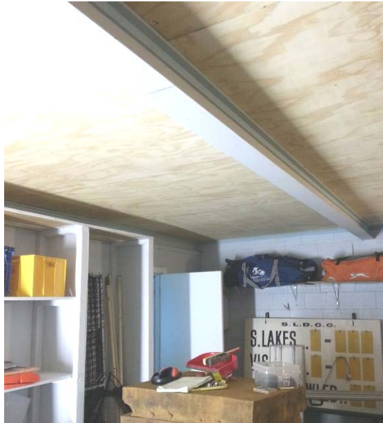
Part of the ceiling in the home changeroom showing the plywood lining.
